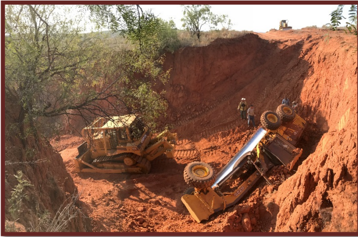
Type I dozer preparing to roll motor grader, looking into ravine from south rim
